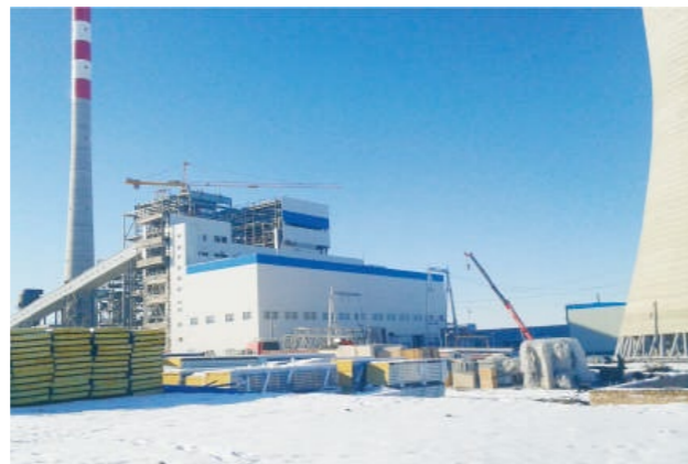
Xingang Power Plant Of Xinjiang 73 Regiment
