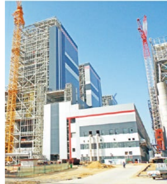
Divine Power China Hami Power Plant
